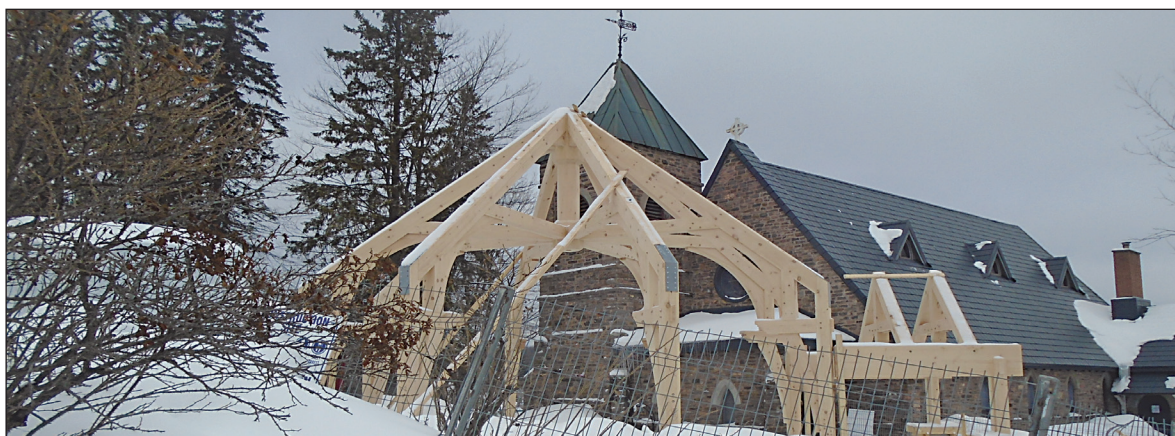
RENOVATIONS UNDERWAY: The construction of a new entrance for All Saints', Huntsville is moving along. There will also be space for an accessible washroom and a meeting and gathering area. The above photo was taken on Saturday, February 11, 2017.
